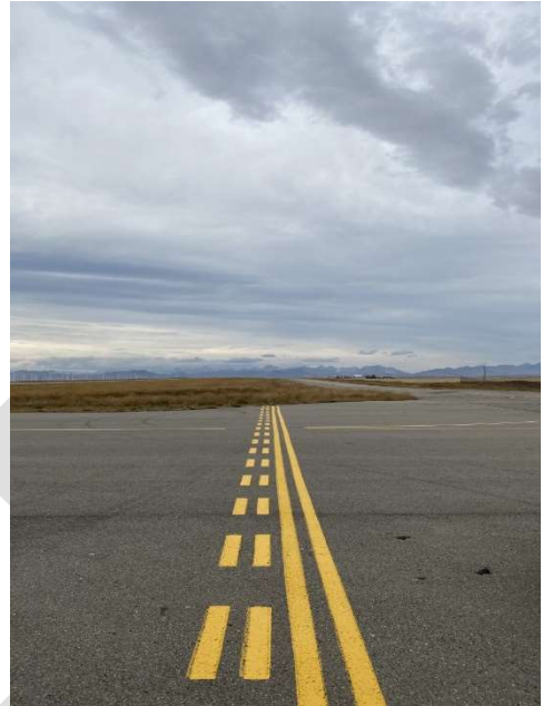
Runway holding-position marking
